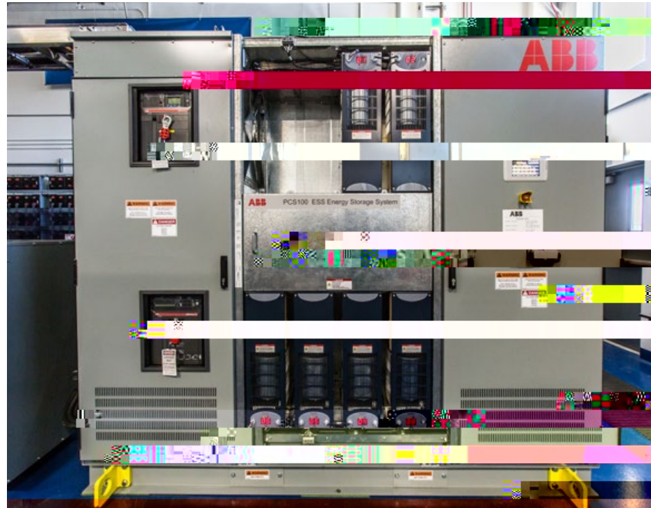
Above: A new ABB Inverter was purchased by ACEP for the testing of Hatch's flywheel system. UAF PHOTO BY TODD PARIS
